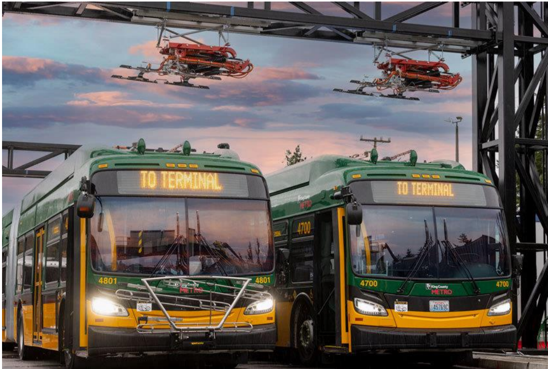
Figure 4: Inverted Pantograph Chargers at King County Metro's Test Charging Facility
