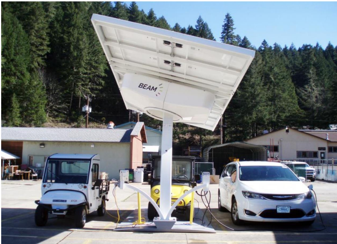
Figure 1. An off-grid solar powered EV charging station
